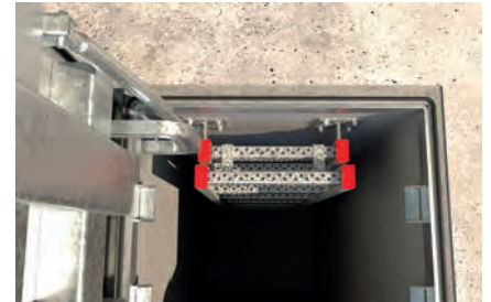
Stormwater overflow tank manholes
