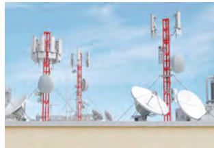
Antenna and masts
